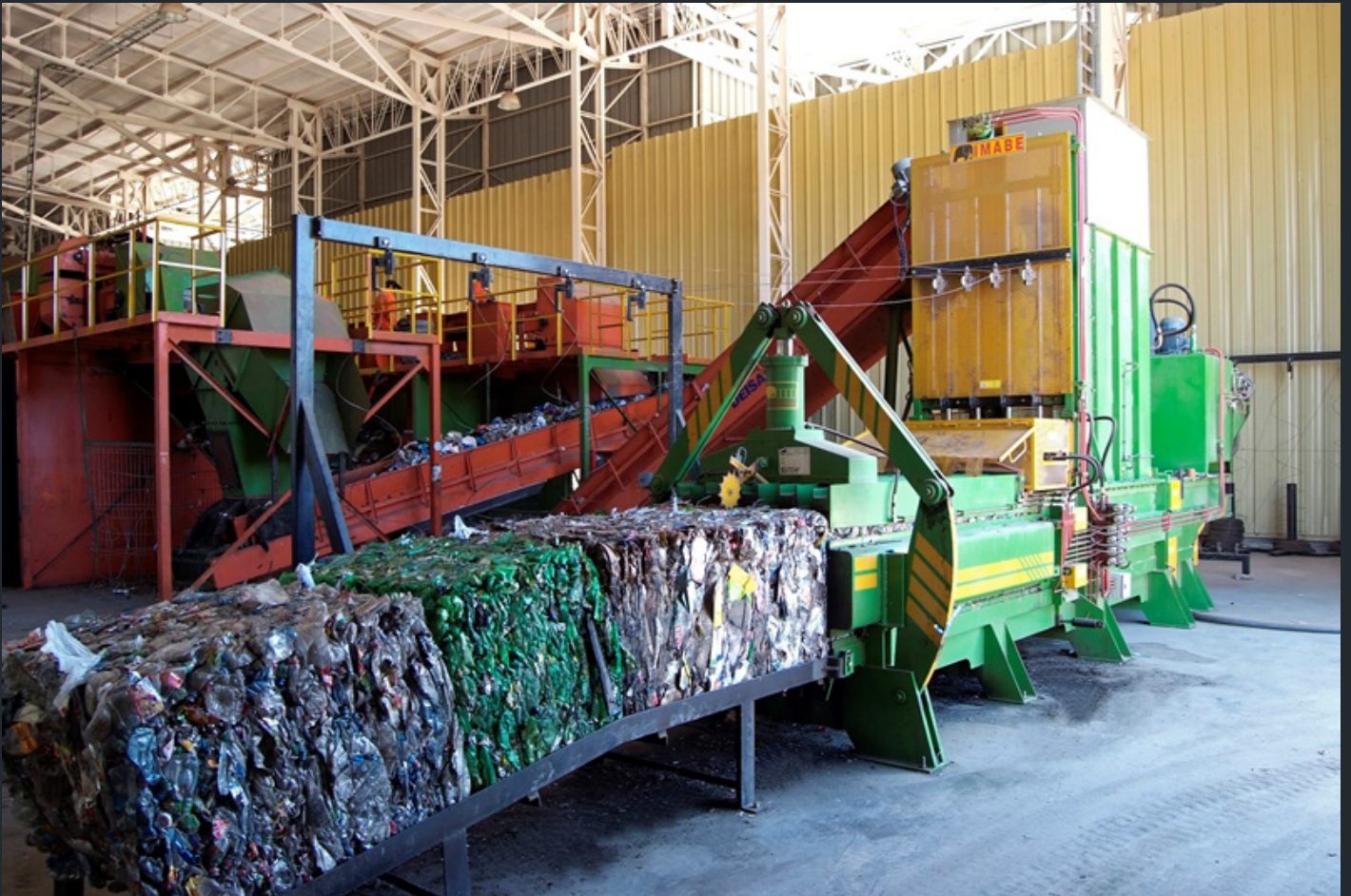
Recycling Plant. Source: Green Tracker
